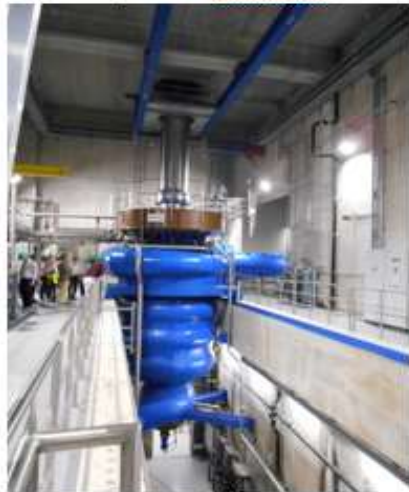
Reverse pump at the Veytaux pump storage installation
