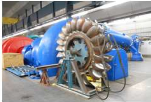
Pelton turbine with spare wheel at Veytaux
